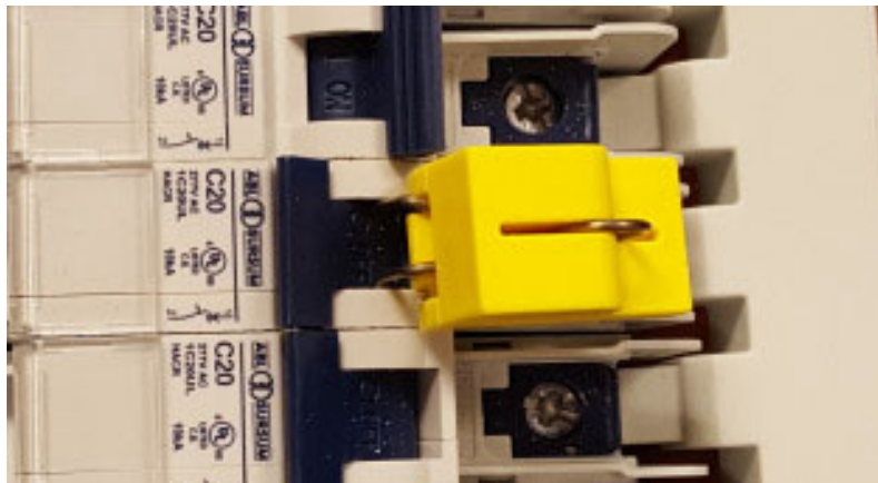
Figure 3.3.1-3 STEP 4: LOCKOUT IN PLACE
